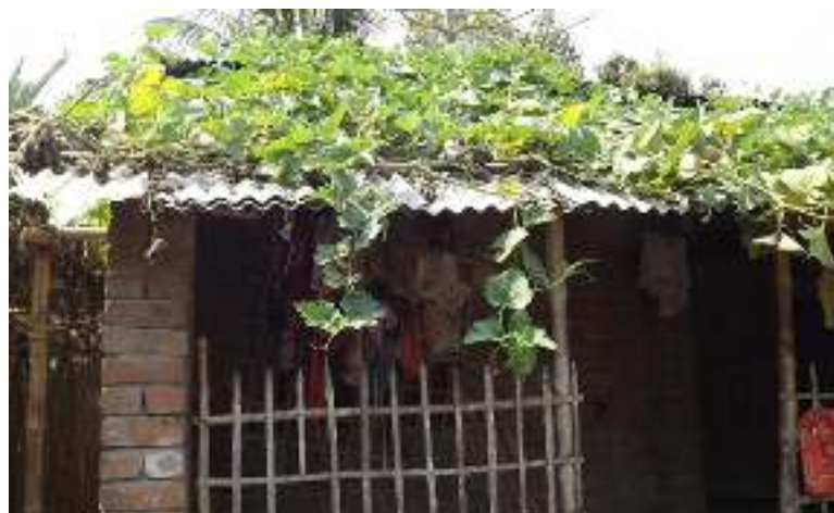
Semi pacca (Brick wall and tin roof) with vegetable production at roof
